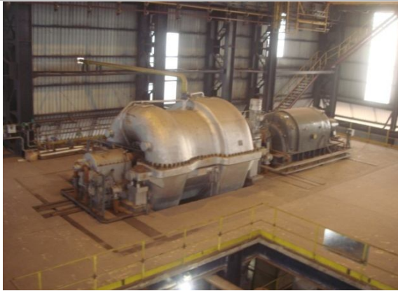
Fig.1. TRT (Top gas recovery turbine)
